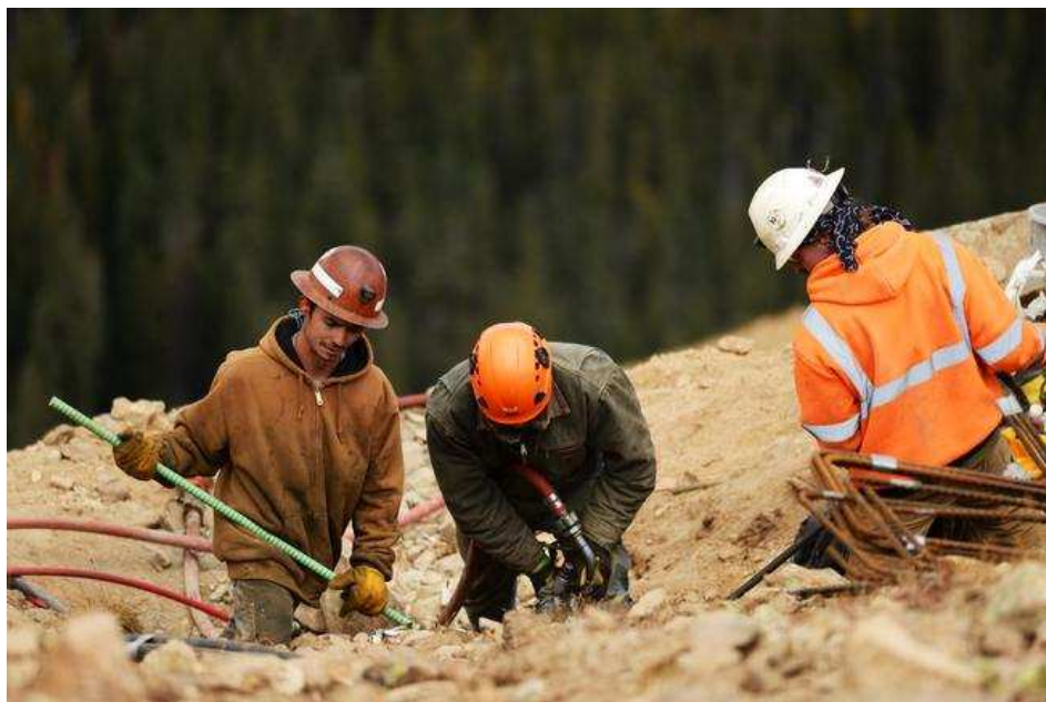
Ground crews are installing the pipes for Gazex Avalanche System at Loveland ski area. ( Hyoung Chang, Denver Post file )
